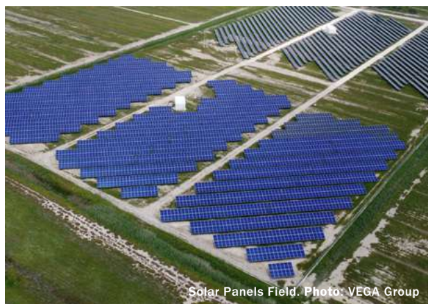
Solar Panels Field. Photo: VEGA Group
